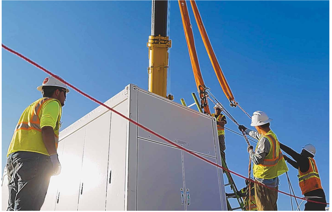
Workers install a battery energy storage container as part of expanding energy storage infrastructure, reflecting growing electricity demand and grid modernization efforts.
